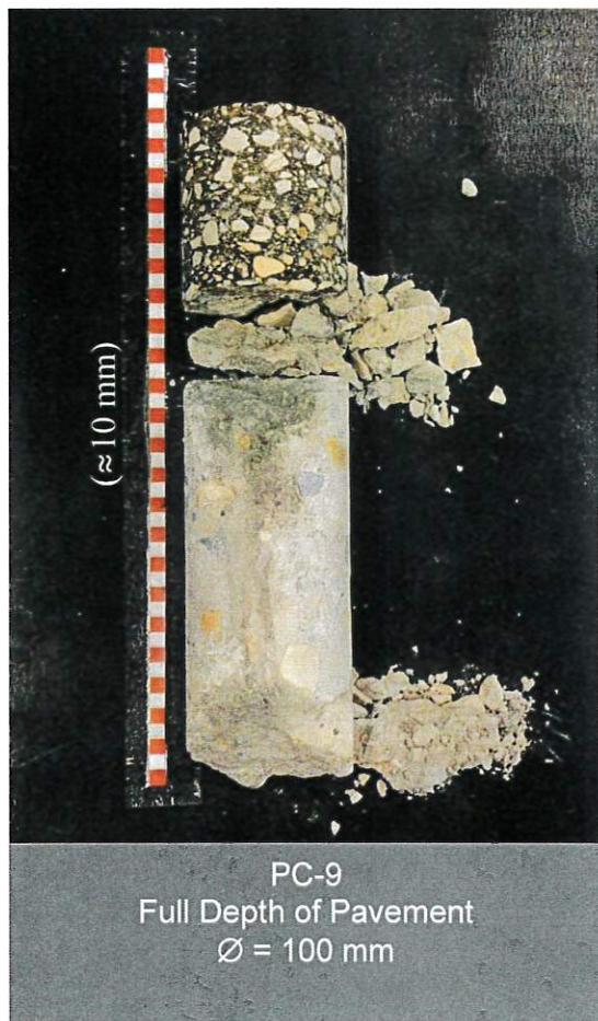
Photograph 9: Specimen from Ellice Avenue, Westbound Curb Lane
